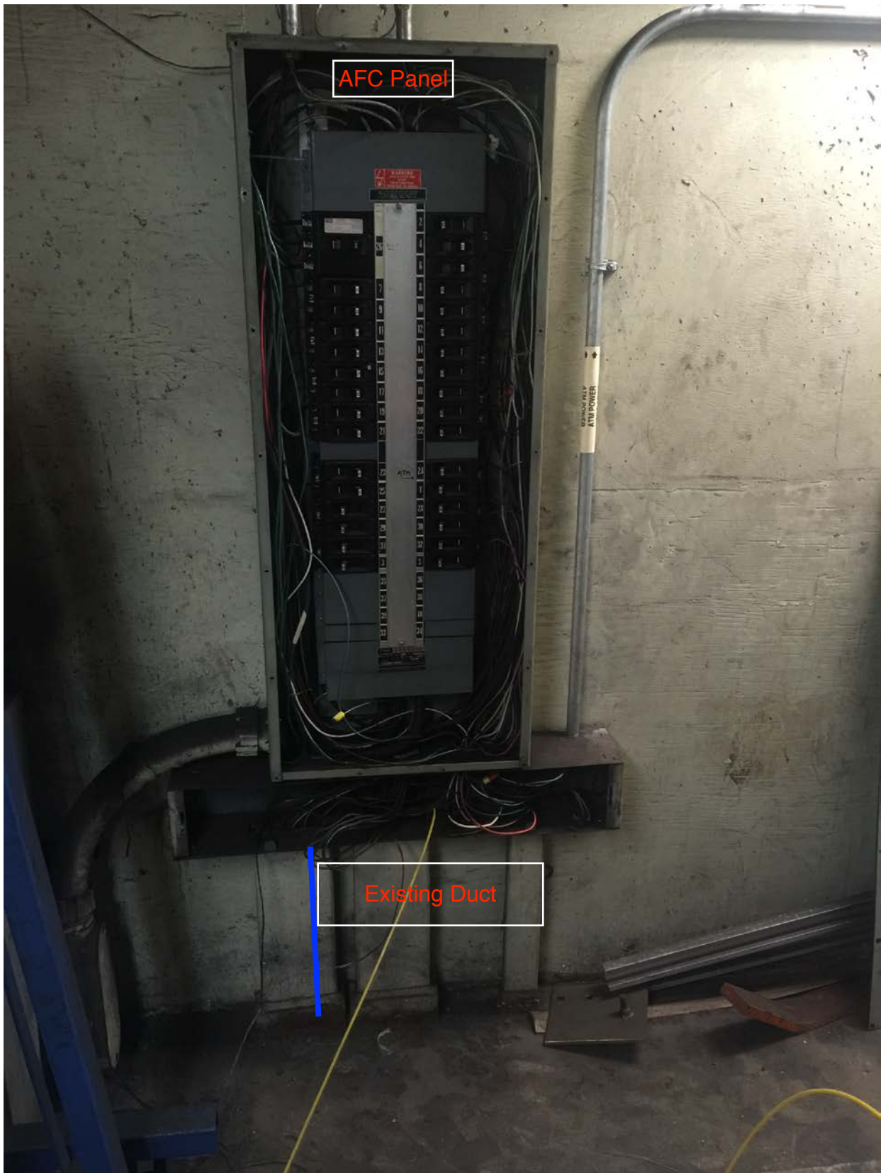
Photo #3 - AFC Panel and duct connection in Room N206.
